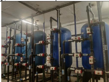
Wastewater Treatment Plant (Activated Carbon Filtration Units) (Yeditepe University, Turkey)
