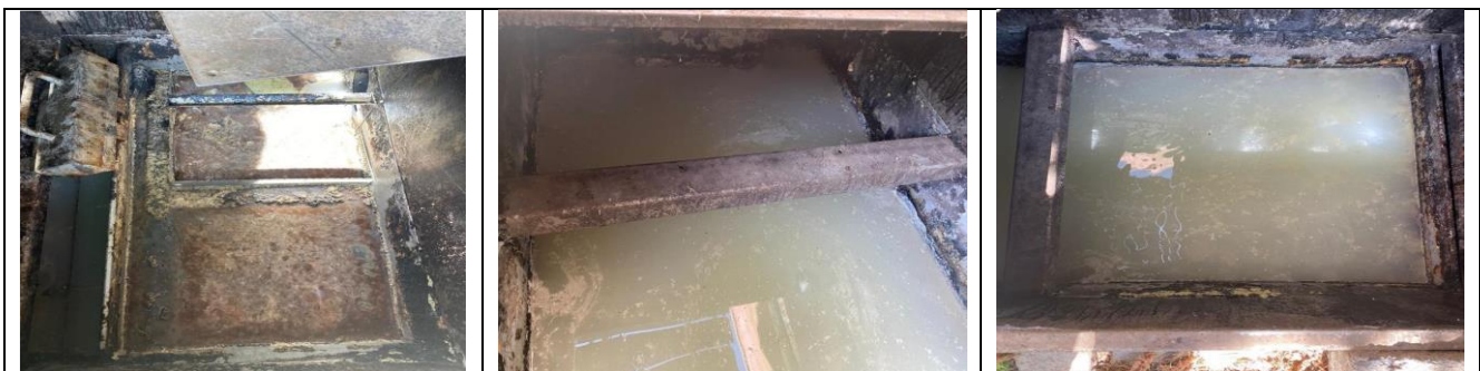
Grease separator tank (Yeditepe University, Turkey)
