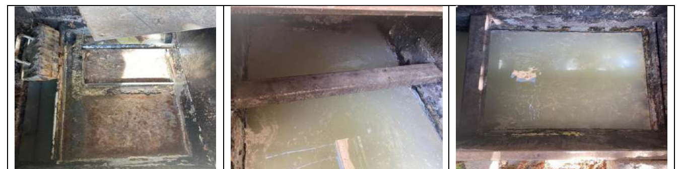
Grease separator tank (Yeditepe University, Türkiye )
