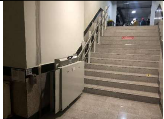
Lifts with disability platforms (Yeditepe University, Türkiye)
