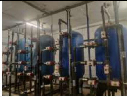
Wastewater Treatment Plant (Activated Carbon Filtration Units) (Yeditepe University, Turkey)
