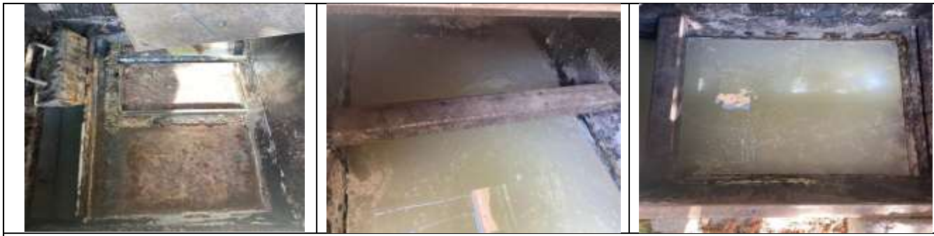
Grease separator tank (Yeditepe University, Turkey )
