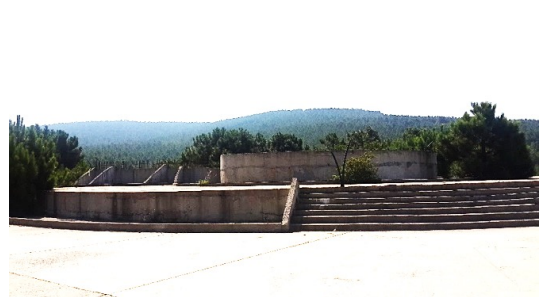
Ground Water Tank in Arboretum Area ( Yeditepe University , Turkey)
