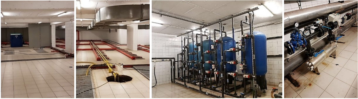
Sewerage Disposal (Yeditepe University, Turkey)
