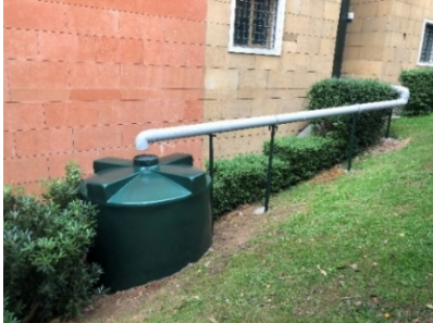
Water Conservation-Rain Water Tank (University of Yeditepe, Turkey)
