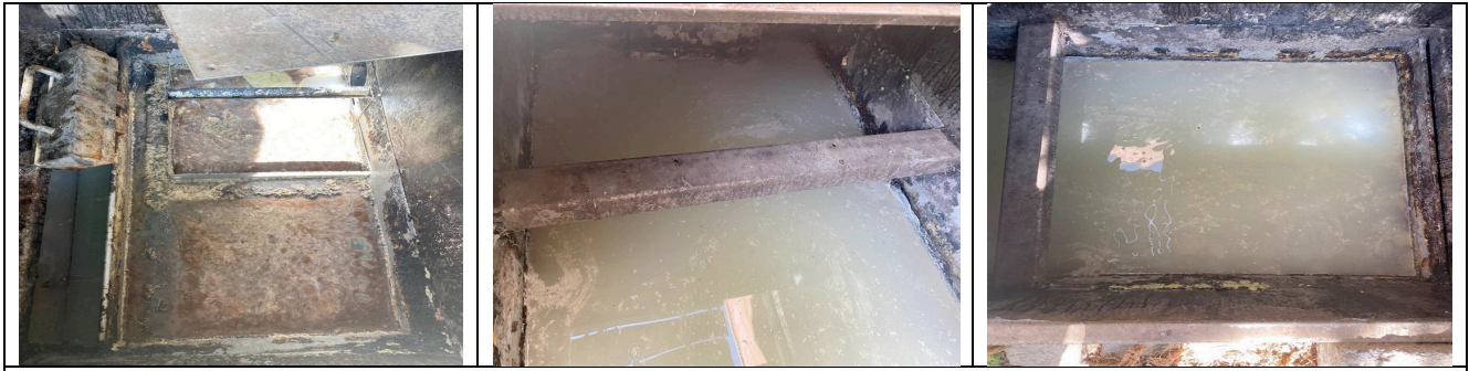
Grease separator tank (Yeditepe University, Turkey )
